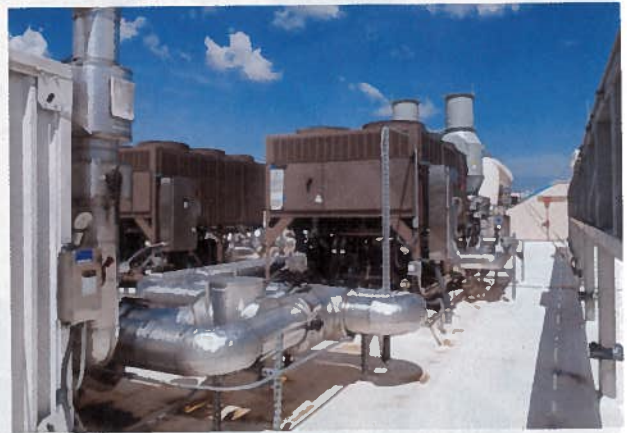
The multifunctional rooftop contains ice storage, chillers, and laboratory exhaust fans.
